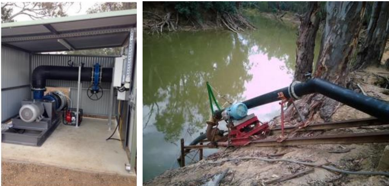
Figure 91 – Irrigation diversion pump stations (Left = Little Murray River, Right = Lower Goulburn)
