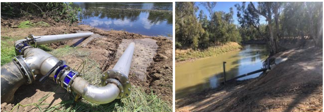
Figure 93 – Examples of Parks Victoria compliant pump arrangements
