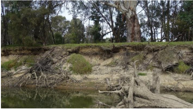
Figure 97: Bank erosion on the Murray River at Brimin (photo courtesy of P Noble)
