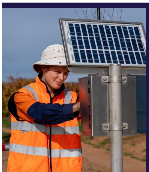
Figure 4. Water corporation field staff reading non-urban meter with fitted telemetry (Woorinen, Victoria).
