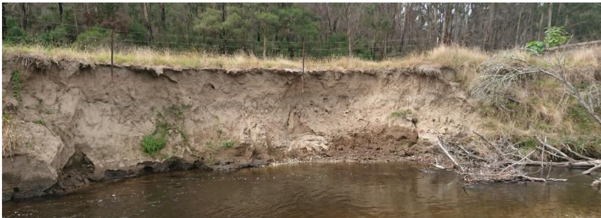
Figure 84. Example site meander bend showing near vertical bank comprised of unconsolidated sands. The fence has been undermined due to bank retreat on Errinundra River.
