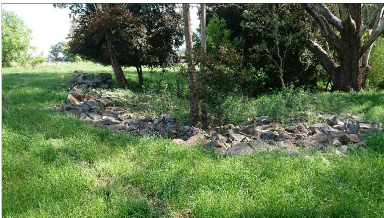
Figure 32. Rock work installed at the upstream end of a developing floodplain channel that conveys flow from the Ovens River (parent channel) to Happy Valley Creek (daughter channel).
