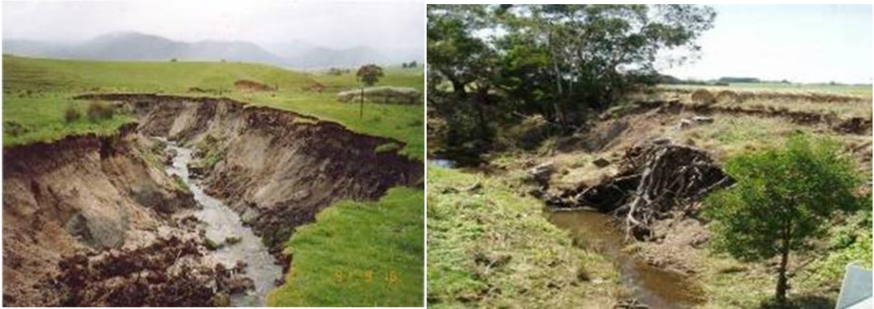
Figure 9. Waterway bed incision, Barwidgee Creek catchment, north east Victoria (left); Waterway bed incision, Mathews Creek, near Deans Marsh, south west Victoria (right).
