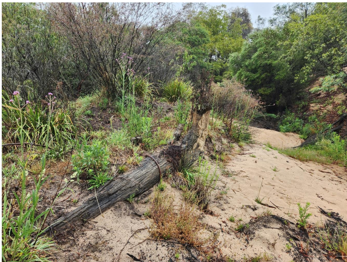
Figure 31. Large woody debris installed in the bed of the Genoa River helping create a stable environment suitable for subsequent vegetation establishment.
