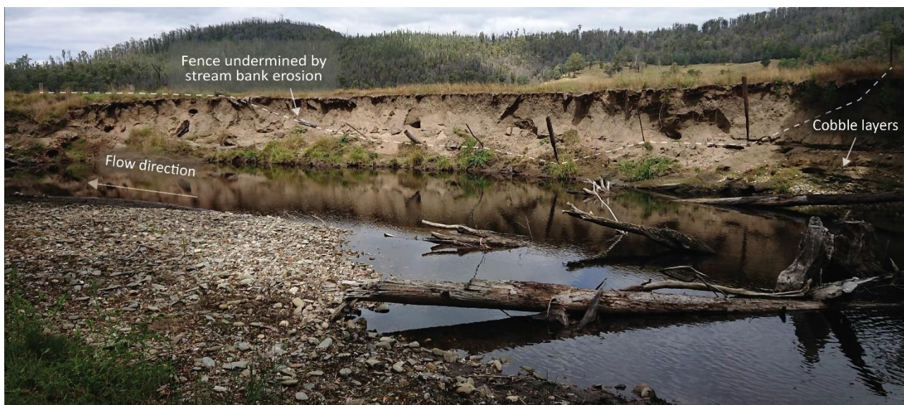
Figure 87. Site 2 – looking downstream, showing near vertical upper bank largely devoid of vegetation. The fence has been undermined due to bank retreat (2021).
