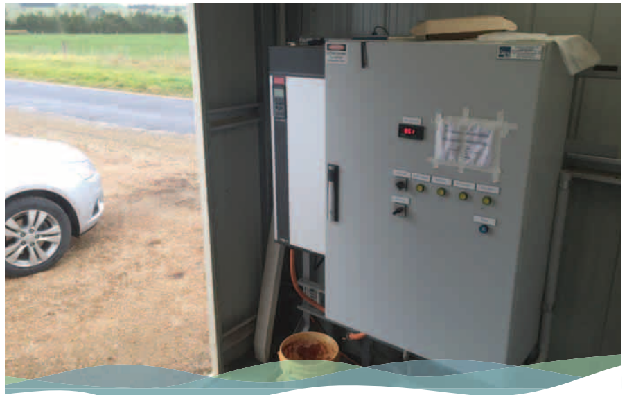
Aquifer storage and recovery bore shed. Courtesy: East Gippsland Water
